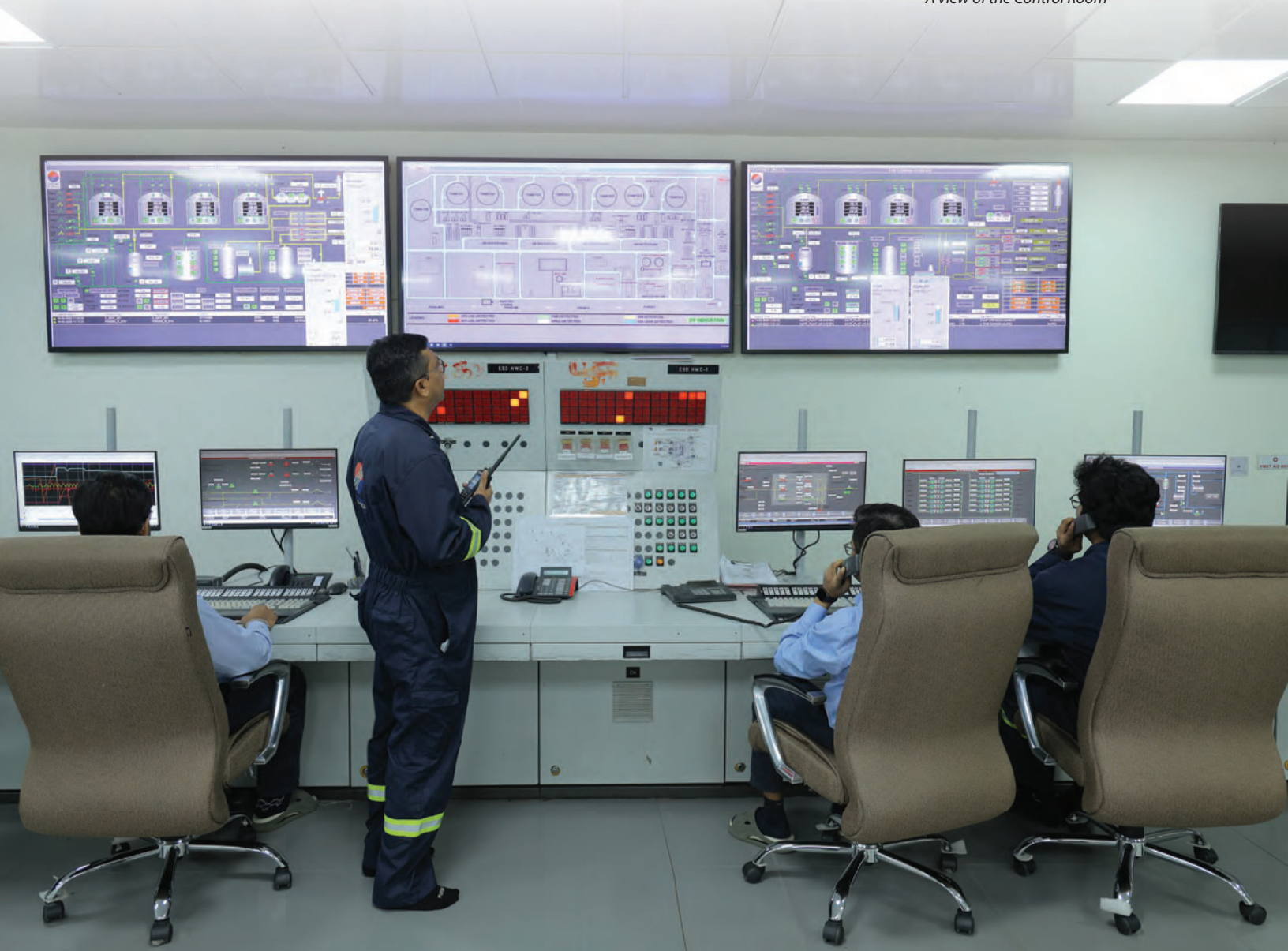
A view of the Control Room
